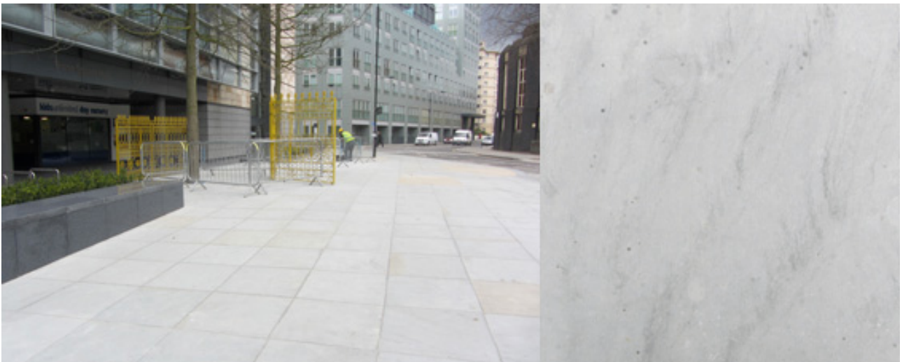
Left: Longford Square. The planter on the far left is Blue Lanhelin Granite with paving of pale grey Whitworth Stone. Right: Whitworth stone showing black flecks of organic matter concentrated along fossil ripples, FOV 30 cm.
