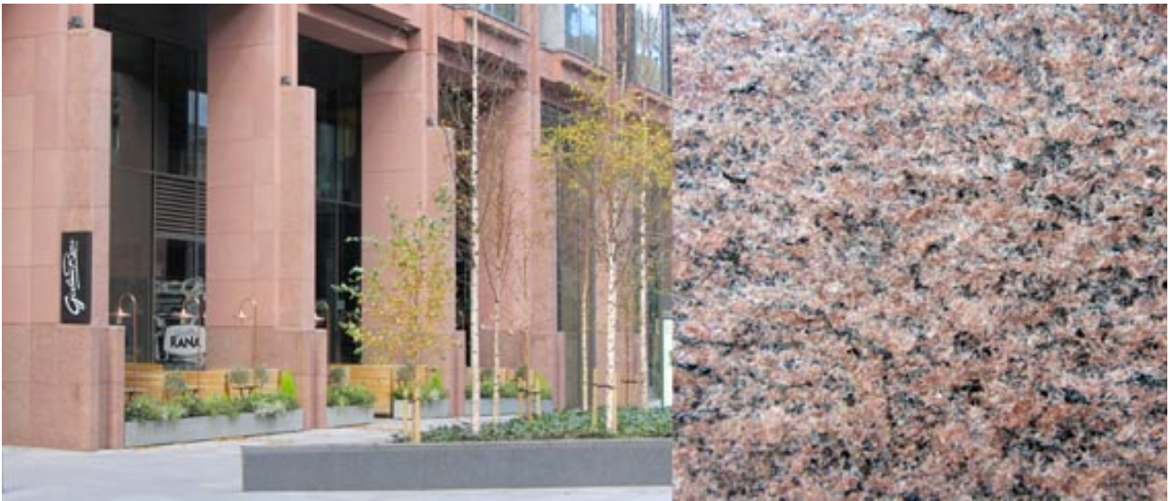
Left: 20 Triton Square, the red granite is at pavement level. Right: close up of the granite, FOV 5 cm.
