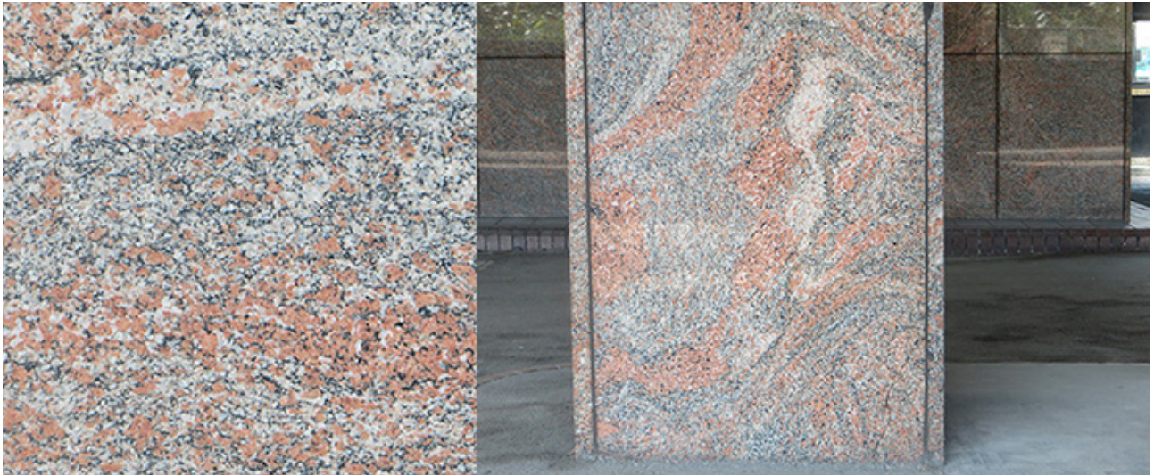
Above left; detail of Parys Gneiss. Above right, contorted Parys Gneiss cladding one of the supporting piers of Irongate House.
