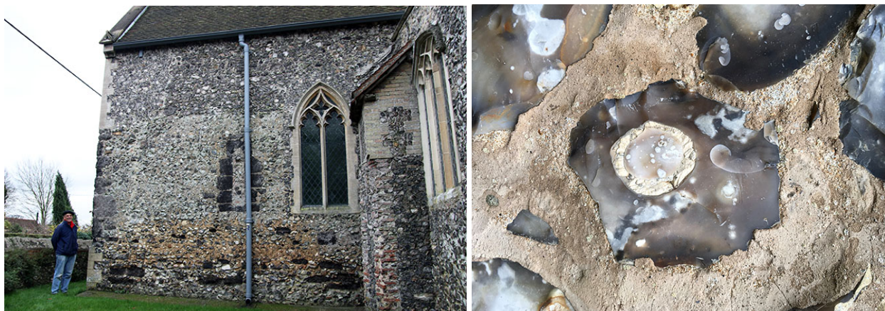
Left: North facing wall of St Peter's Church, Belaugh showing several phases of construction and restoration and the distinctive, almost black blocks of ferricrete. Right: Knapped flints from the south facing wall containing a Conulus sp. Echinoid.
